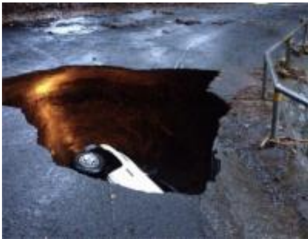
A flooding storm at the end of 2013 undermined a road culvert and swallowed a truck and driver on Pohakea Mauka Rd. CERT helped in this emergency.
