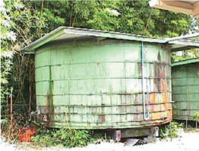
An older redwood tank. Beware of redwood tanks that were painted on the inside with lead paint to discourage algae.
