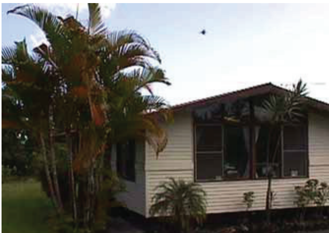
Do not allow trees and bushes to overhang your roof. They provide roof access to rats and other vermin.
