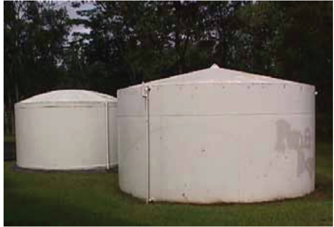
These enclosed metal tanks are well maintained on the outside, but problems may arise if there is deterioration on the inside.
