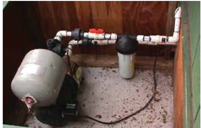
A small but typical electric pump. The pump sits below a pressure chamber. A coarse filter hanging from the inlet pipe filters the water before it enters the house.
