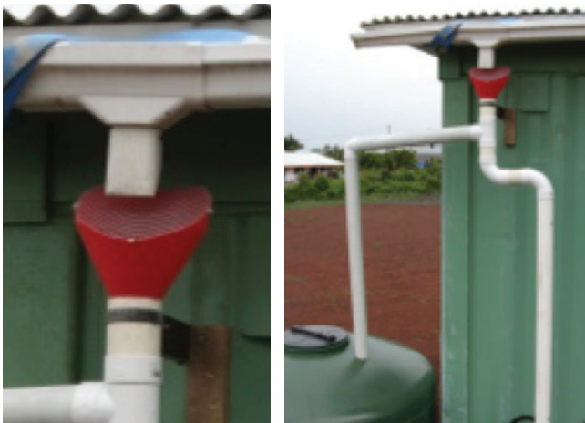
Homemade leaf screens and first-flush diverters can be made inexpensively, such as this one, which uses a large funnel and galvanized screen to keep leaves out and PVC pipe to divert the first flush of water.
